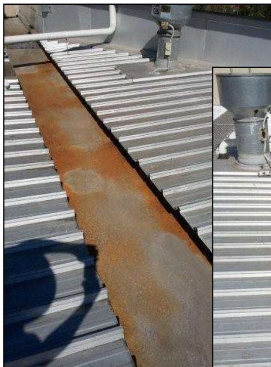
Rusted box gutter corroding and leaking
